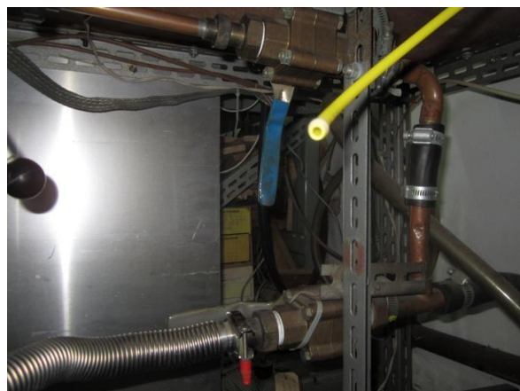
Fig. 2. Hoses, ball valves and bellows used in the 3IPLAP vacuum system.
