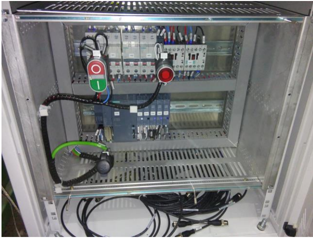
Fig. 1. Front view of one of the two prototypes of the bakeout controllers mounted at the LNLS/CNPEM. Behind the plexiglass front one can see the rails with the CLP modules at the bottom, and the power part, with breakers and solid state relays at the top. On the front one can see the ON/OFF and reset switches, besides the Ethernet port (lower left).
