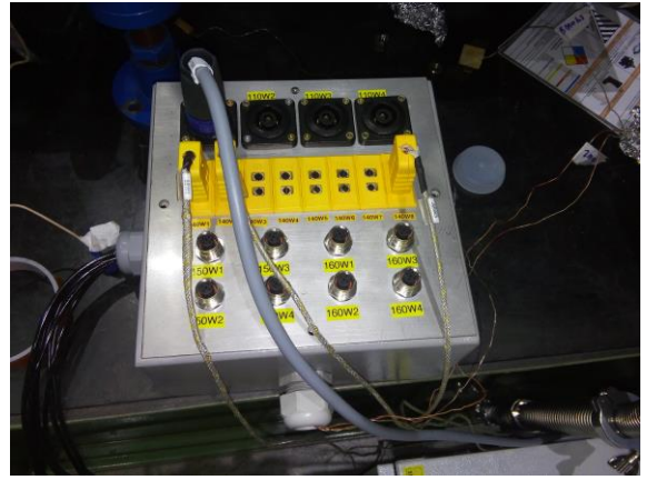
Fig. 2. Distribution box or patch panel, permanently located close to the system to be baked out. The tapes and temperature sensors are connected to the bakeout controller using specific made cables.
